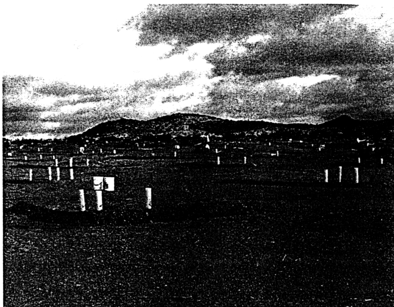
Berm and basin catchment system for the desert. The view from downslope at Fort Irwin, California during construction of catchments the authors designed to funnel surface-runoff water into planting areas. In these trials, catchments increased survival of some species planted inside collection areas, but results depended on size and design of the simple berm structures, which must be adapted to rainfall, slope, soil permeability and other factors. Photos by authors
