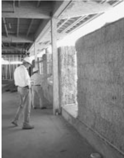
Wall installation at the Santa Clarita, Calif., bus facility. (Photo by Rick Green, who grew the rice straw bales and supervised the installation)
