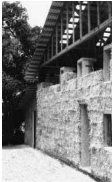
At Tree of Life Nursery the pole and roof were put up first, allowing the wall construction to proceed safely as a potential rainfall threatened.
