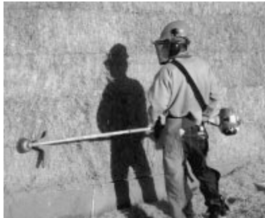
The bale wall is trimmed before plastering at a Santa Clarita, Calif. bus facility. (Photo by Rick Green)
