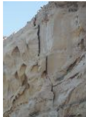
Torrey Pines Crack 2014 -this flake fell the following year
